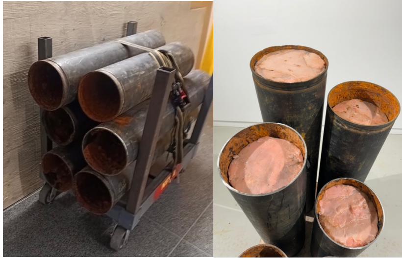
Figure 36. Pipe pedestals, extracted from OCAD foundry ventilation system, February 2025. Photos by author.
