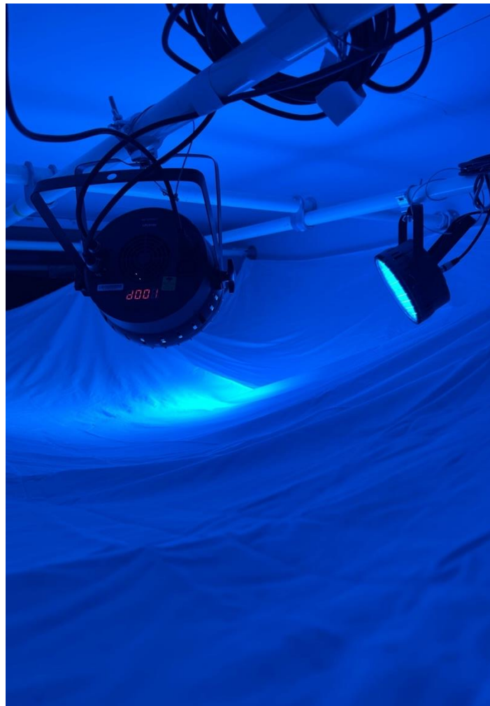
Figure 41 Prototype 3, DMX-Controlled Par lights allow for the installation space to be completely immersed in colourful light, (Figure by author, Toronto, December 2025).
