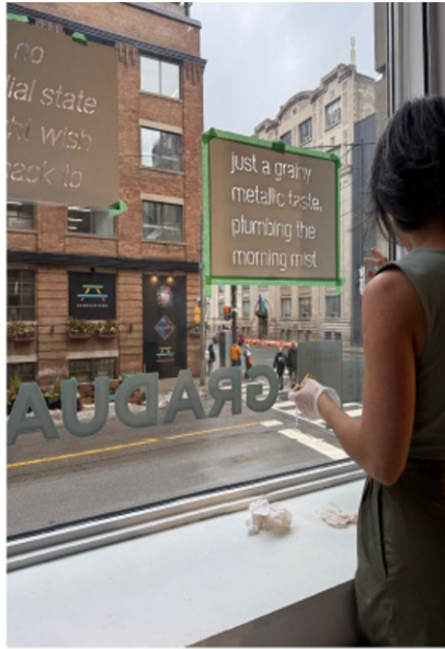
Figure 10. Installation of the poem from Footnotes for an Arsenal 2022, 2002 . by Dana Prieto Photo D. Bosco
