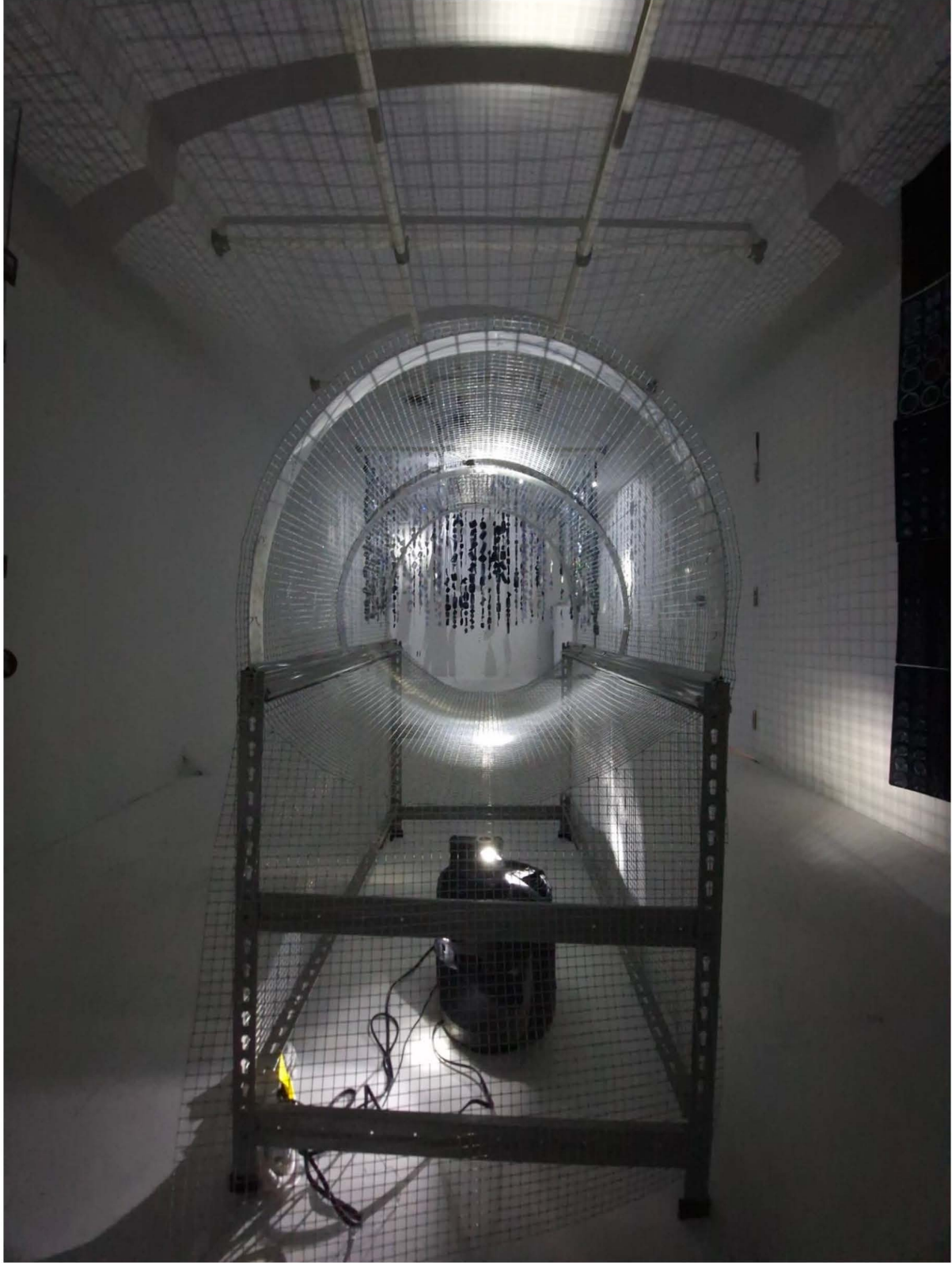
Figure 32: MRI Installation - Number 9
